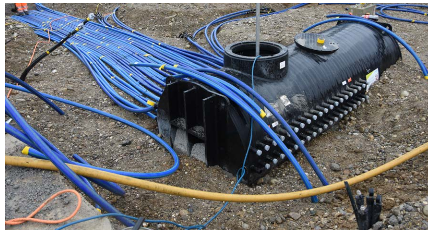
Nine JANSEN u-boot underground distribution shafts were used. The cylindrical, horizontal submarine-shaped distribution shafts offer sufficient space for large distribution dimensions, special installations and up to 80 brine circuits.
