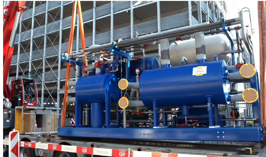
The large heat pumps from the Swiss manufacturer Walter Wettstein AG provide a total of around 5.5 MW of heating and cooling power. Each machine is six meters long and weighs 15 tons. They are operated with the natural refrigerant NH3 (ammonia). When designing the probe field, the energy requirement was estimated at about 5 to 6 GWh per year.
