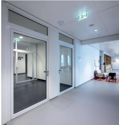
pic 02: Airlock between the rental area (two single-leaf doors)- and the lift vestibule (double-leaf, "permanently open" door there)
